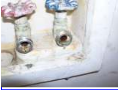
Washer valve actively leaking
