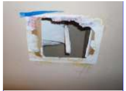
Missing toilet paper holder
