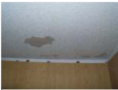
Texture missing in garage
