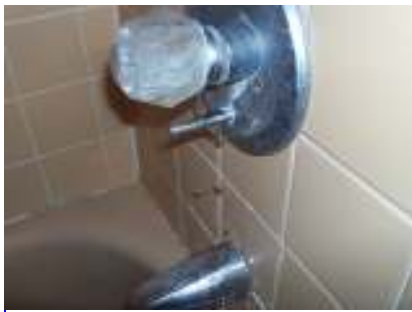
Hall bath faucet handle leaking
