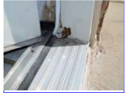
Front door wood rot in jamb
