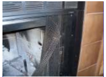
Broken fireplace screen
