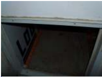
Air handler missing filter
