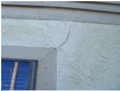
East side large settlement cracking
