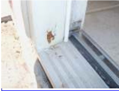
Front door wood rot in jamb
