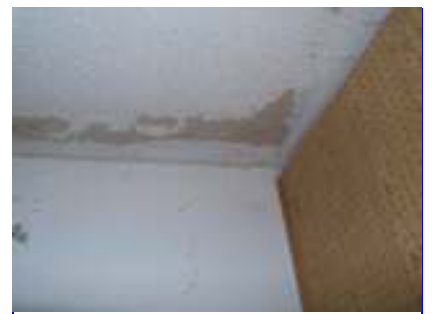
Texture missing in garage
