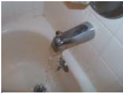
Master faucet "stuck" on shower
