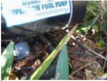
Pool pump leaking and not working
