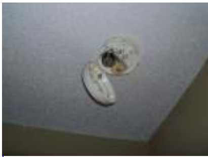
All smoke detectors are broken
