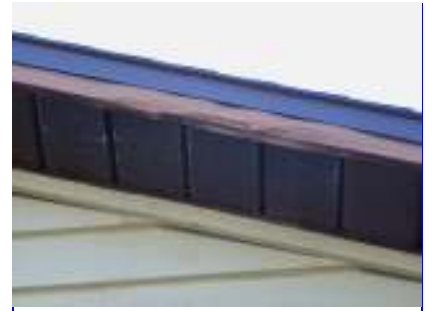
Crumpled fascia on East side
