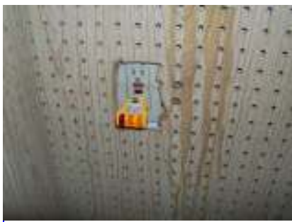
Garage GFCI malfunctioning
