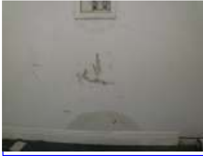
Water damage to wall in laundry
