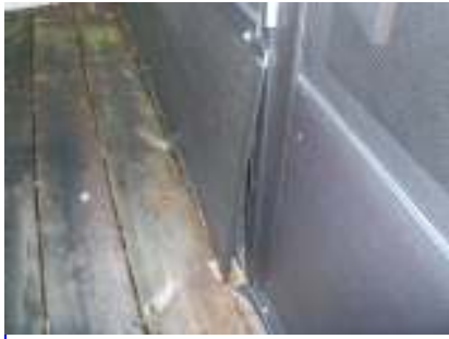
Screen room kickplate loose
