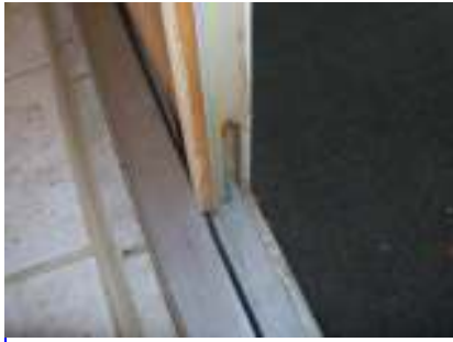
French door slide lock missing
