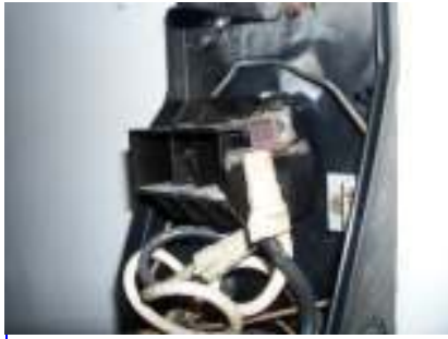
Air handler disconnect broken
