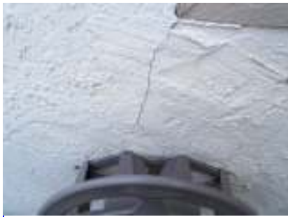
East side large settlement cracking
