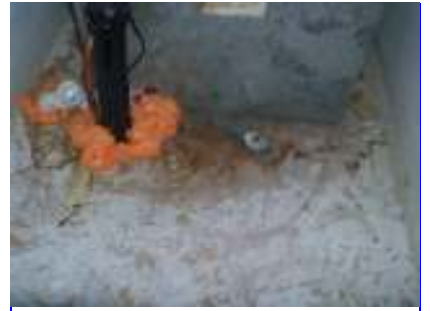
Previous water damage on base
